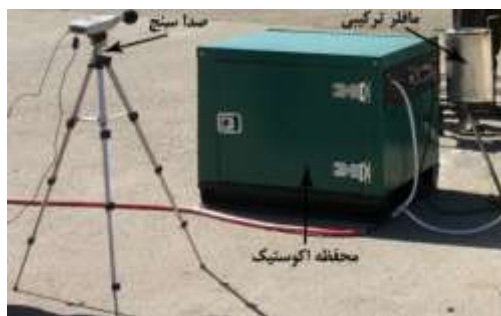
Figure 3. Gas Genset with reactive muffler covered by acoustic enclosure and sound level meter.
