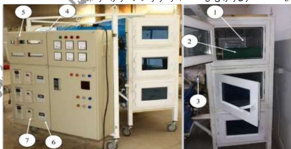
Figure 1- Semi-industrial continuous dryers used to dry tomato slices: 1) drying chamber, 2) conveyors, 3) heating elements, 4) radial fan, 5) electrical panel system for controlling temperature and air velocity, 6) thermostat, 7) Inverter.
